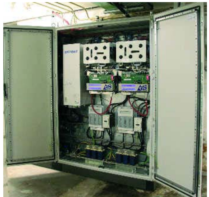
Fig. 8: AS-frequency controller PM/PD 1000 Converter – The first built Papermachine-Profi-Drive – Converter from AS
